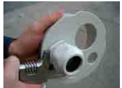
3. Connect the screws with the pipe fairlead and fix the screws
